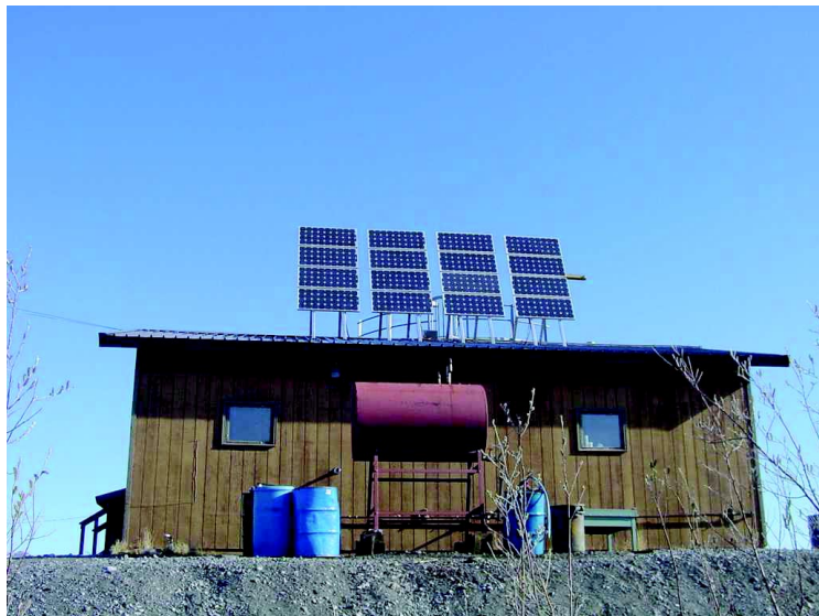
1.2 kW photovoltaic system atop washateria in Arctic Village, Alaska.
